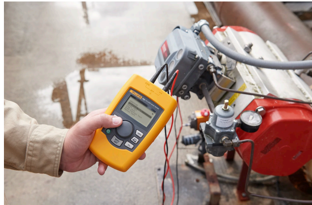
As part of custody transfer, technicians routinely calibrate all the pressure and temperature transmitters involved in the flow of oil & gas
