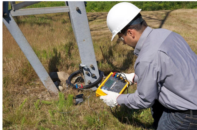
Stable voltage, safe earthing, clean harmonics — the measurable foundation of Syria's rebuilt grid.
