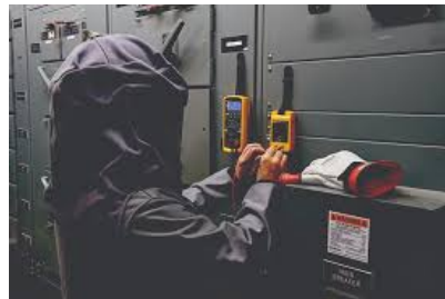
Testing at energised switchgear is carried out under controlled, standards-based safety procedures
