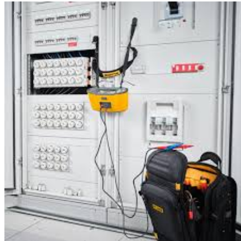
Reliable installation testing is essential for ensuring the safety, and optimal functionality of a facility's electrical systems.
