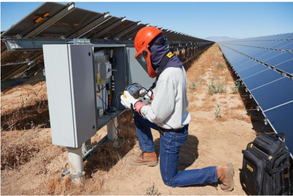
Performance verification relies on accurate field measurements to IEC 62446 and IEC 61724
