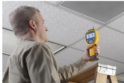
Testing the air upstream and downstream verifies that filtration systems are capturing contaminants as designed.
