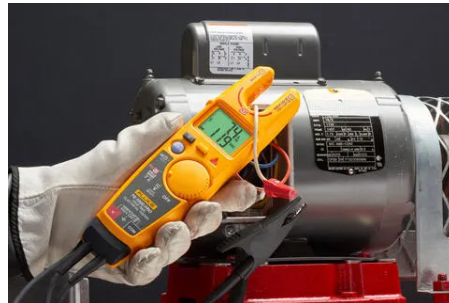
Field measurement verifies generator output and protection against rated values
