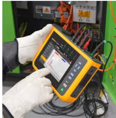
On-site logging measures real consumption patterns across each major system
